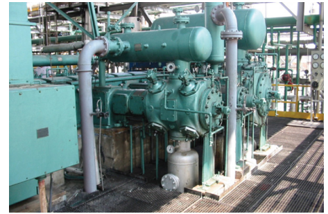
Booster and primary compressors
